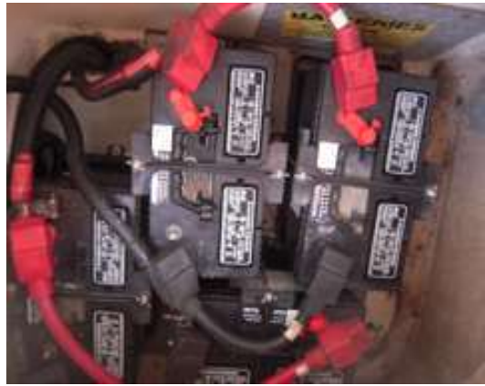
Batteries, secured and protected
