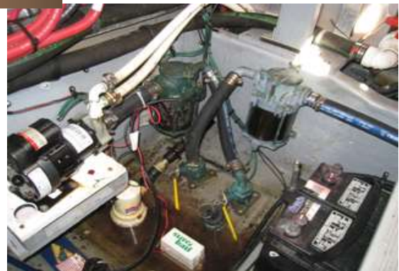
Potable water pump and misc equipment
