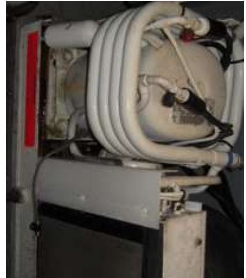
One of two air/heat units
