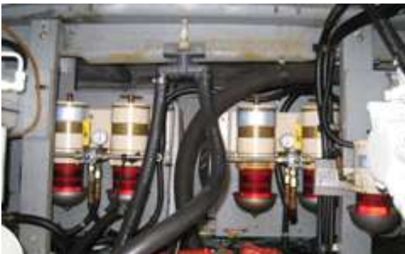
Fuel supply and filters
