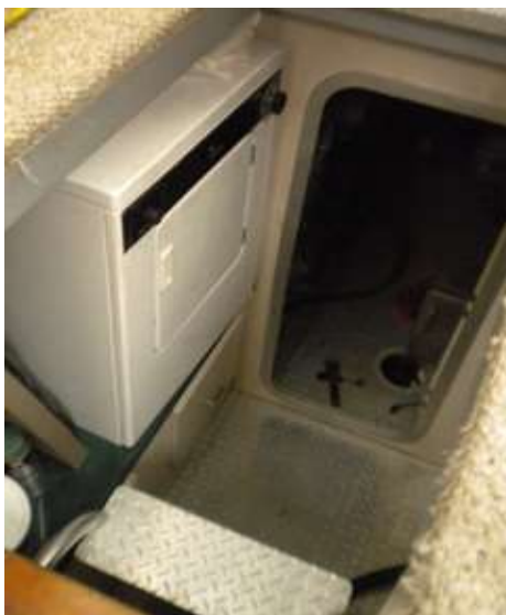
View of full size clothes dryer, a new washer is being installed
