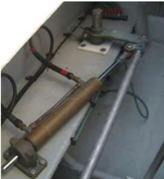
This image shows good working hydraulic steering gear
