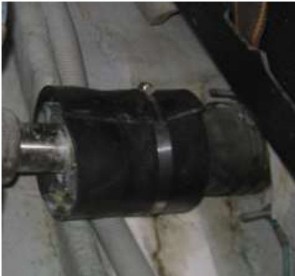
This image shows water cooled shaft log and clean bilge.
