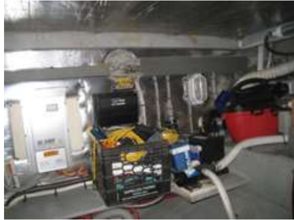
This image shows wanother septic system hose that is in need of service.
